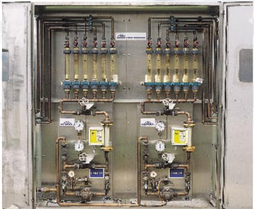
Oxygen measurement and control unit
