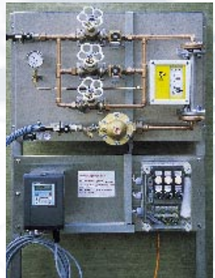
Oxygen measuring and control unit with electrical switch box
