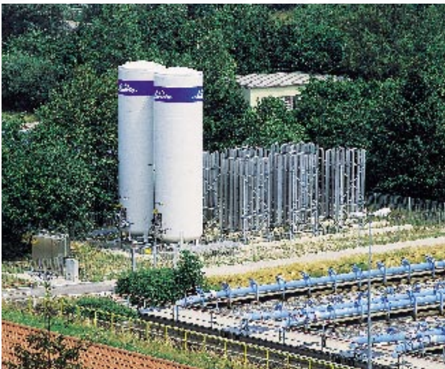
Oxygen supply plant
