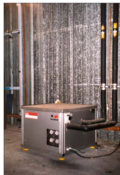
Liquid CO 2 pump system
