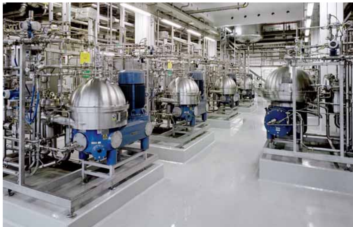
A view into a large-scale biopharmaceutical plant, designed and constructed by Linde-KCA-Dresden.
