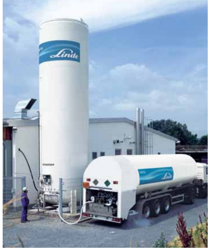
Bulk delivery of liquid nitrogen.
