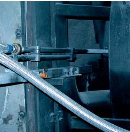
WASTOX® lance in a single-pass furnace
