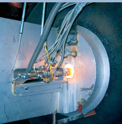
WASTOX® lances in a double-pass furnace
