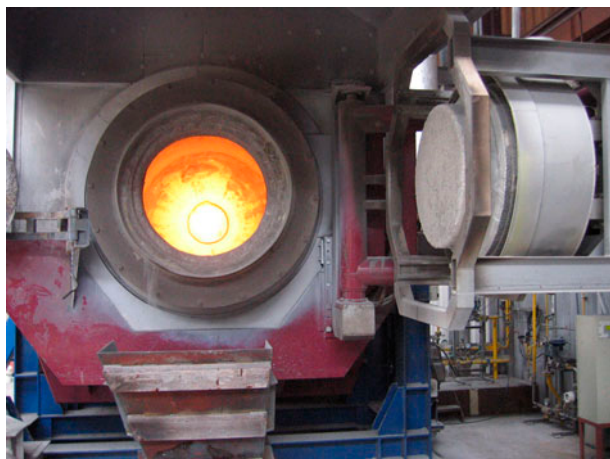
Fig. 5: AluMonte melting furnace with bouncing shield to control overpressure inside the rotary furnace.
