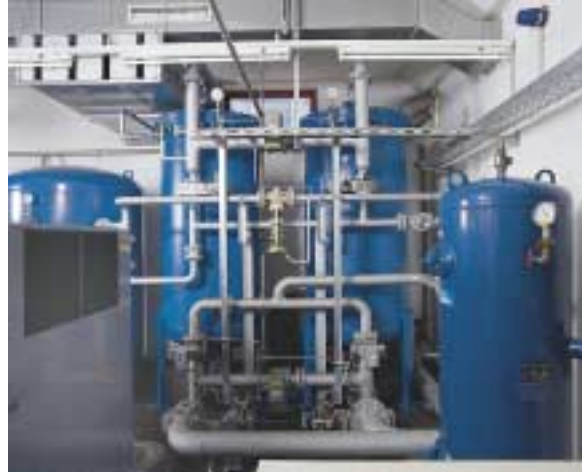
View of a PSA plant with a capacity of 300 Nm 3 /h nitrogen
