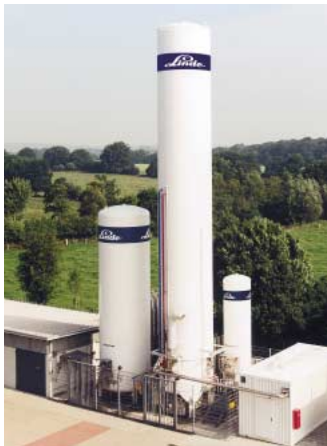
View of a cryogenic plant with a capacity of 600 Nm 3 /h nitrogen
